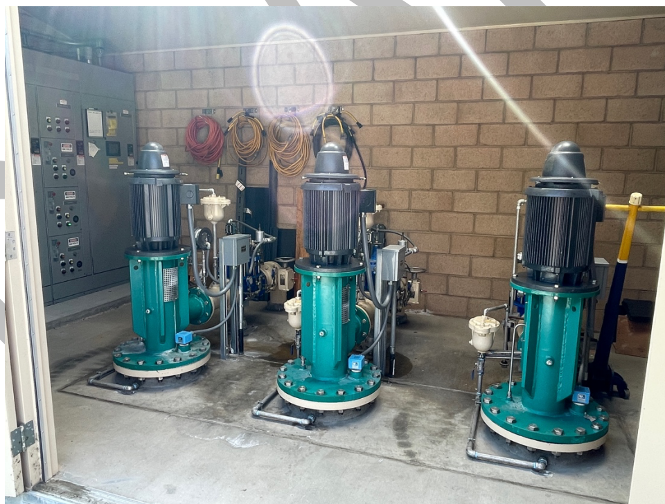
Figure 2-22. Vosburg Booster Pump Station View 2
