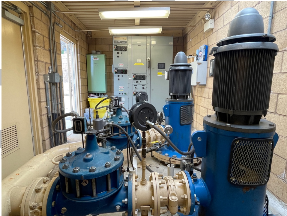
Figure 2-17. Sage Booster Pump Station View 2
