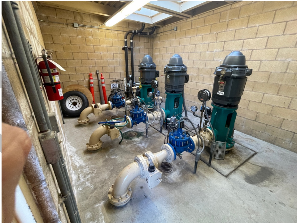
Figure 2-15. Eucalyptus Booster Pump Station View 2
