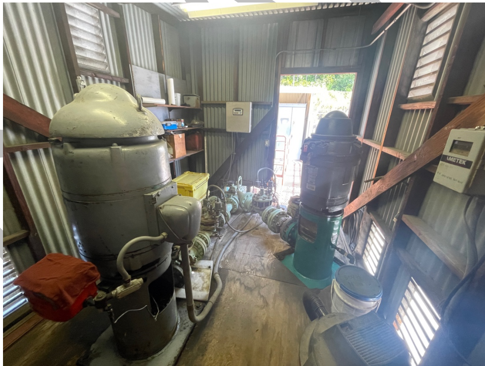
Figure 2-19. Wilcox Booster Pump Station View 2
