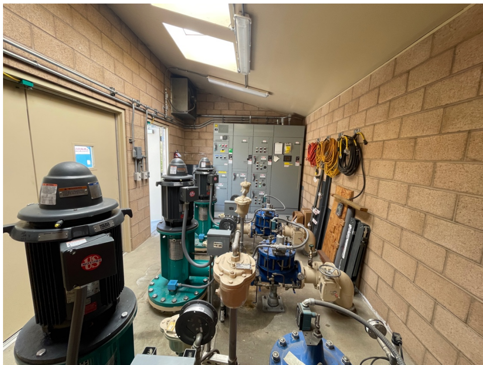
Figure 2-21. Vosburg Booster Pump Station View 1
