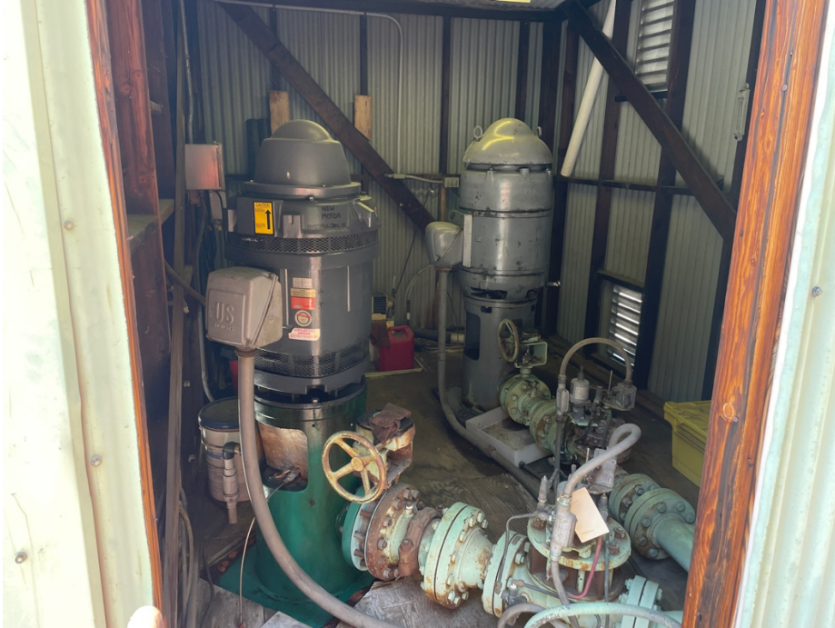
Figure 2-18. Wilcox Booster Pump Station View 1
