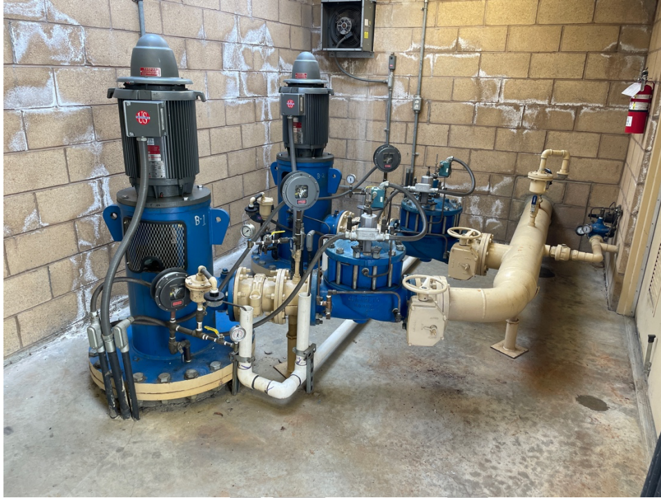
Figure 2-16. Sage Booster Pump Station View 1
