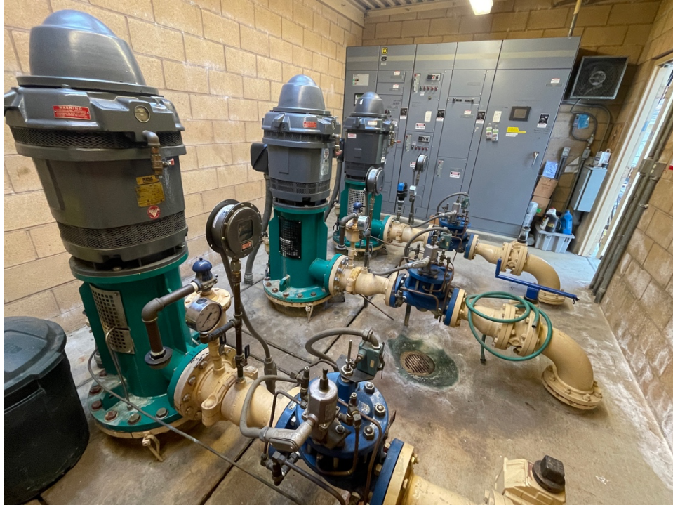
Figure 2-14. Eucalyptus Booster Pump Station View 1
