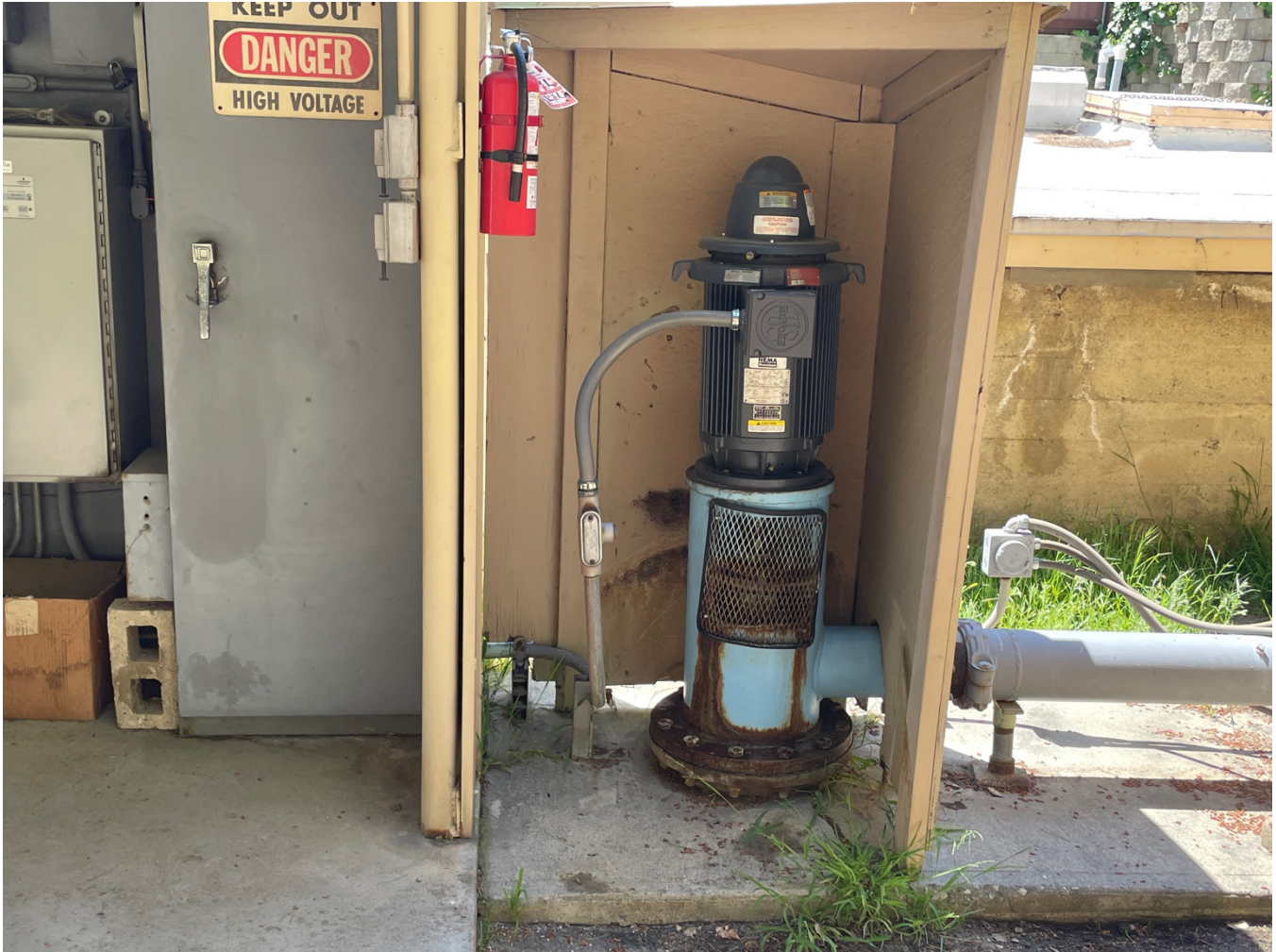
Figure 2-20. Glen Booster Pump Station
