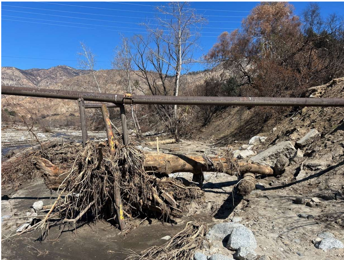
Close up photo of damaged pipe support and coupling.
